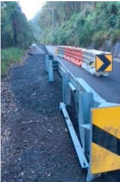
Below: The same section in 2022 after further deterioration & temporary repairs
