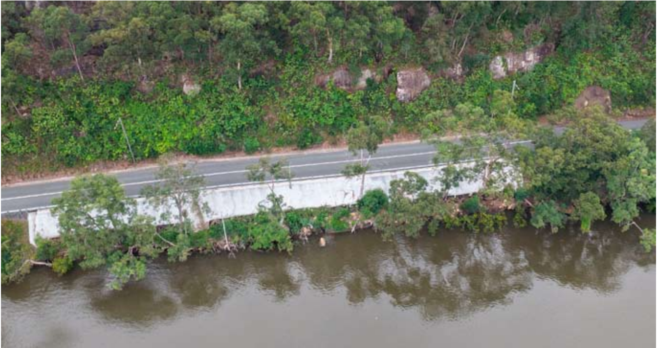
Above: Restoration at Gunderman - Back to two lanes after almost 20 years! The embankment rebuilt and stabilised
