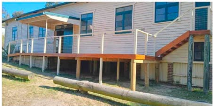
Top: The old deck and stage exit stairs Bottom: The new deck and stairs
