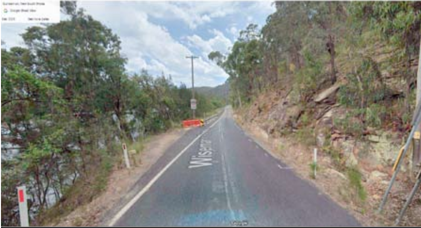
The section of Wisemans Ferry Rd at Gunderman that is included on Council's Capital Works interactive map. This section had partly collapsed many years ago..
