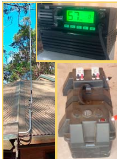
Left: Antenna, Top Right: CB and power supply, Bottom Right: Backup battery
